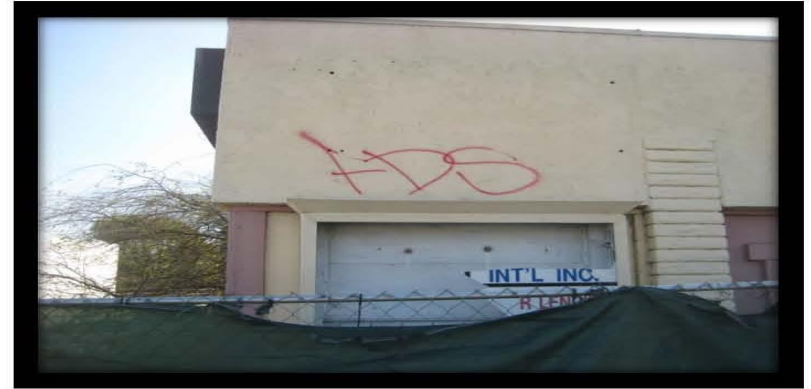
Excessive vandalism & broken sign
