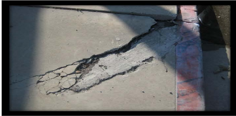
Cracking of the sidewalks
